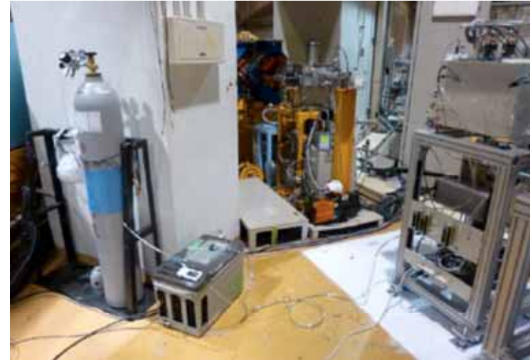
Gas pipes to bottle & ref.
