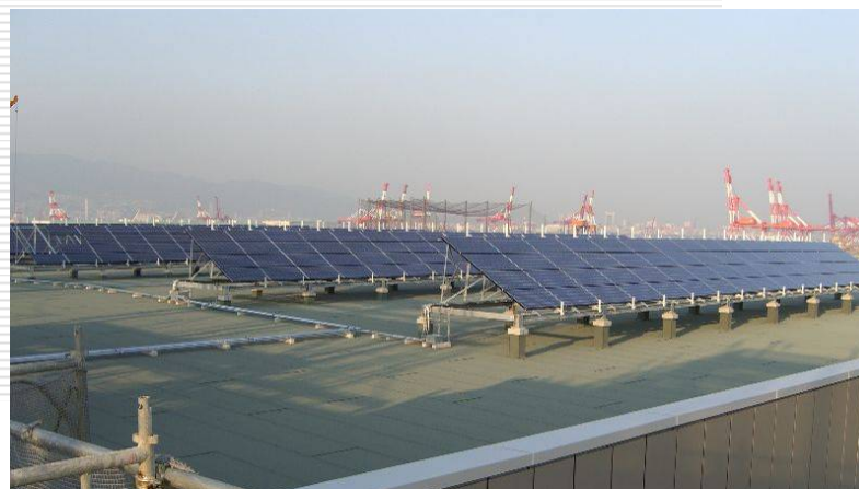
Solar panels on the top
